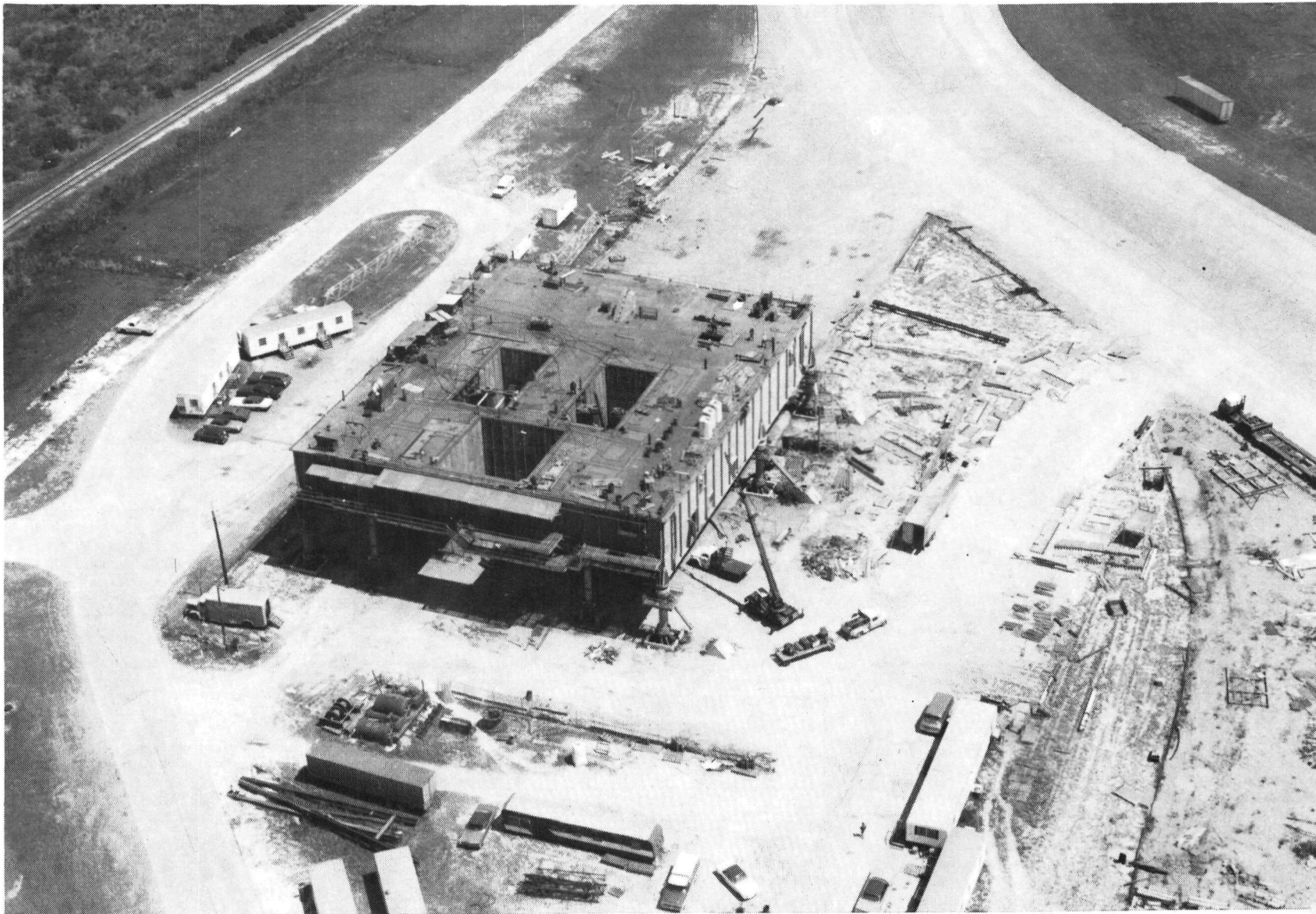
Figure 7 -- The Apollo mobile launcher undergoes major modifications to fit it for transporting the Space Shuttle vehicle. Most obvious changes include three "flame bucket" openings instead of the previous single aperture. Umbilical towers have also been removed from the mobile platform.
